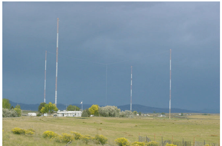
WWVB's four north towers supporting the broadcast antenna wires in the center. Credit: NIST
