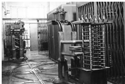
Photo: A temporary railway was used in the construction of Daventry, and a more permanent system - complete with 'points' - was used to move 'trucks' carrying the grid and anode tuned circuits (as shown).
